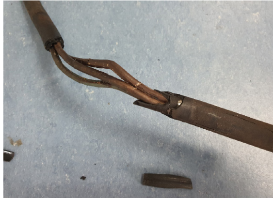
Figure 5: Part of the degraded cable sample
